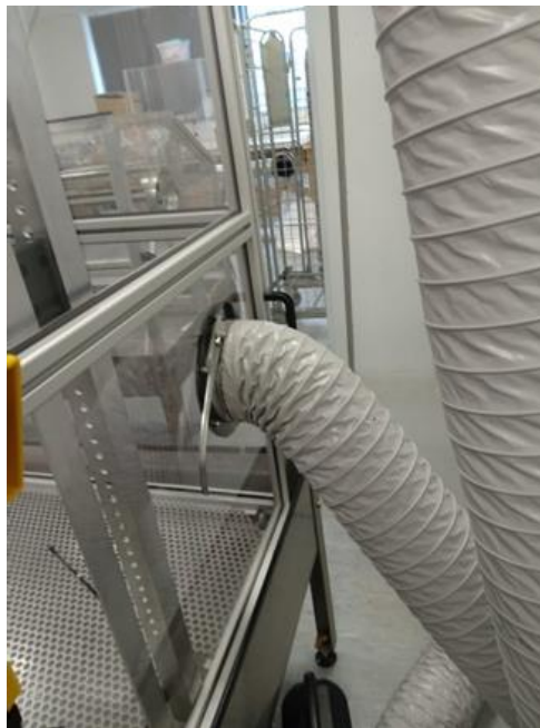
Figure 5: Tubing attached to filtermist and enclosure
